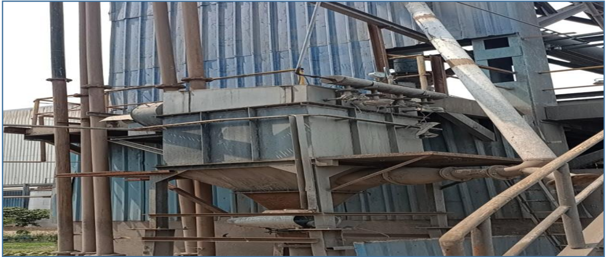
Bag filter for coal crushing section
